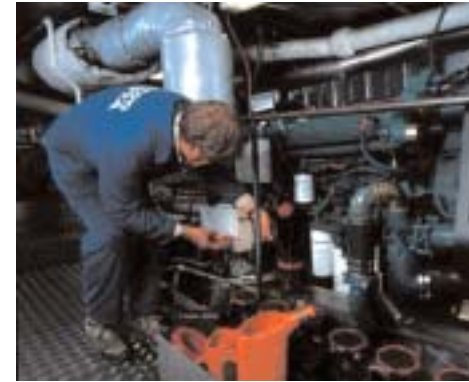
Volvo Penta carries out 'certified installations' to ensure that engines are installed correctly at boatbuilders' premises.
